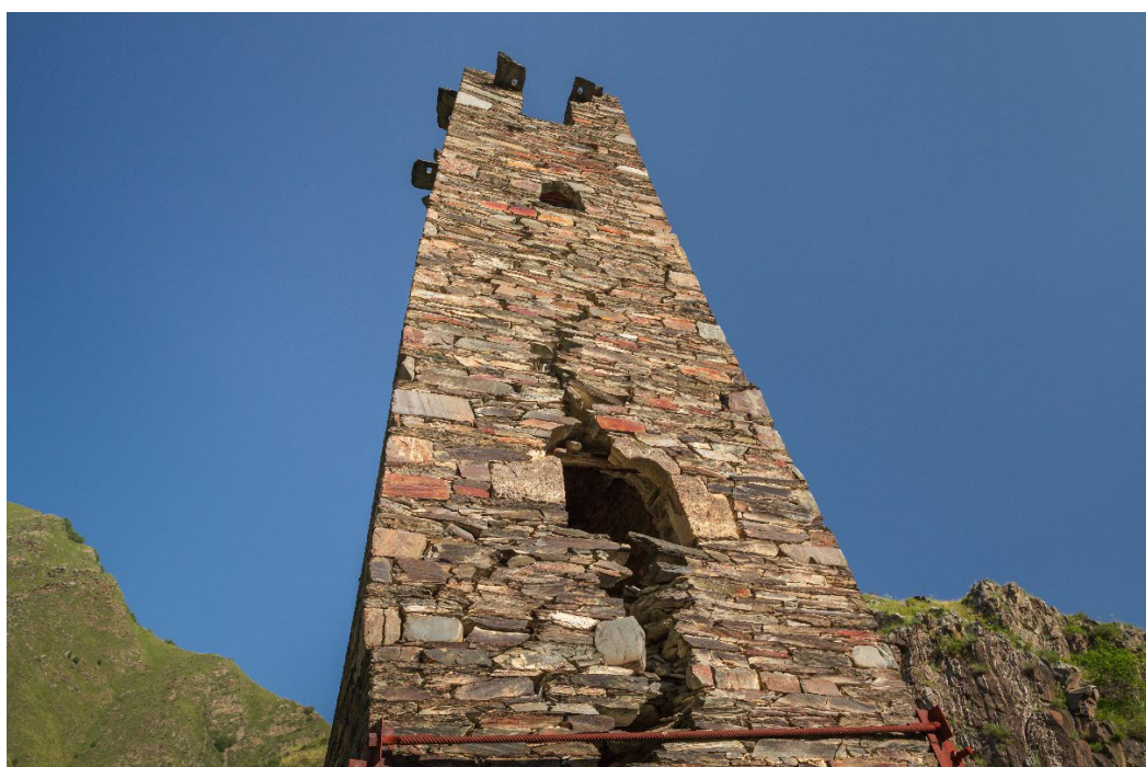
Figure 3. Photo taken in 2017 before repair and restoration
