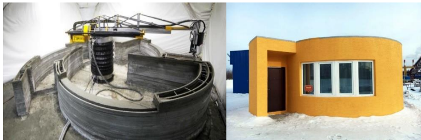
Figure 04. Apis Cor 3D printed house. (Left: building printed; Right: completed house) Source: ApisCor (2017)
